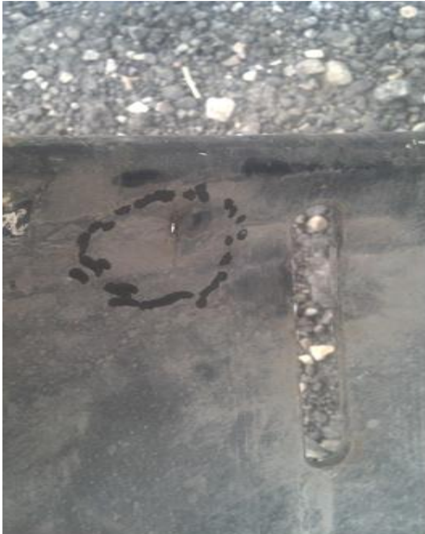
Light through the raised portion of the stop. Not Damage
